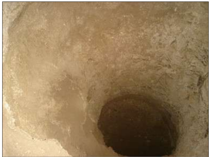
Figure III.19: Rupture de bouchon de catiche rue Émile Zola. Source: GRIMP (ARR285)
